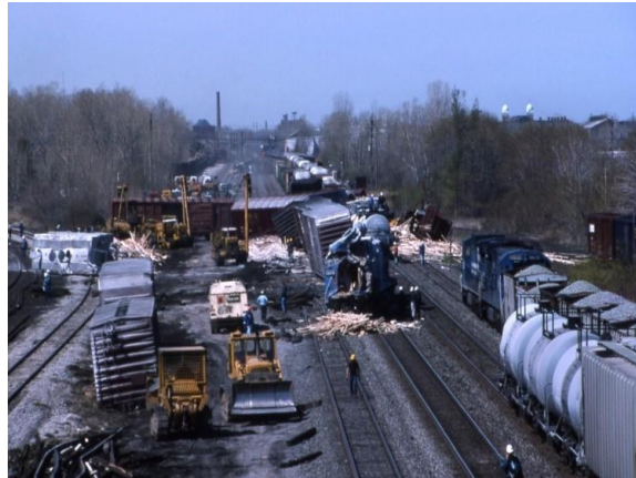
This 1995 derailment in eastside Erie (the twin peaks of St. Stanislaus Church can be seen at upper right) symbolizes the continuing problem that trains face with out-of-date tracks.
