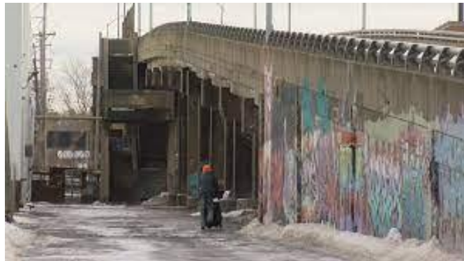
The base of the former McBride Viaduct off East Avenue in Erie
