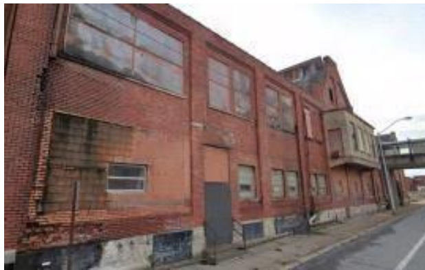
Erie Resistor Corporation building shown in a deteriorating state
