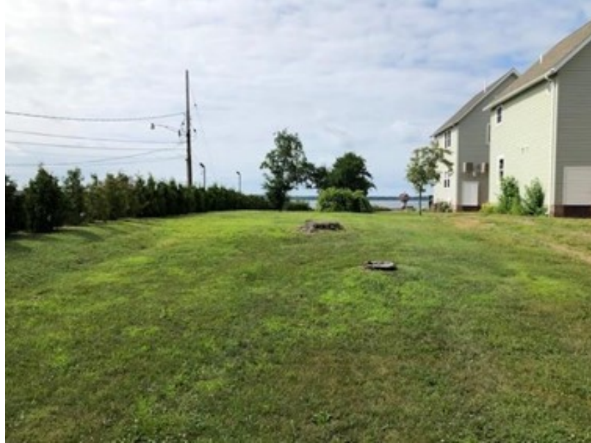
The final vacant bayfront lot is now a construction site where a huge new multi-unit building is taking shape.
